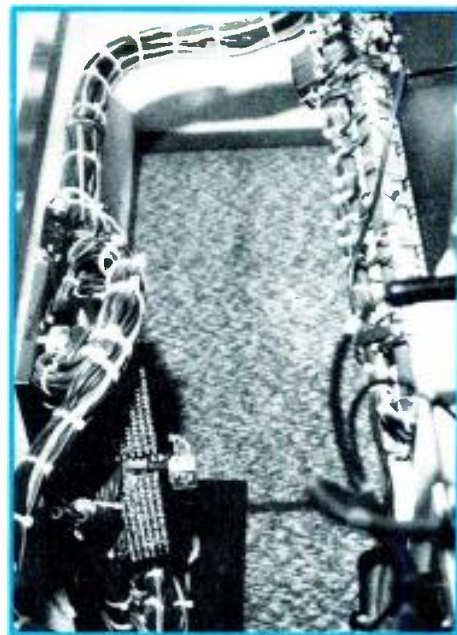
An access path of at least 18 inches should be left behind the control room equipment to allow servicing.
