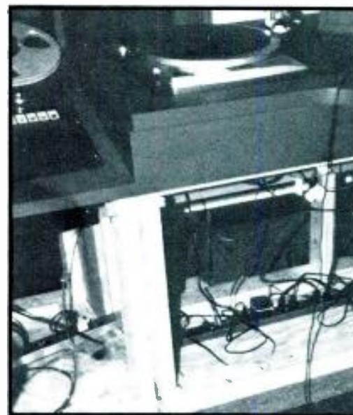
The cabinet panels are quickly removable to reveal the patch bay and hidden circuitry.
