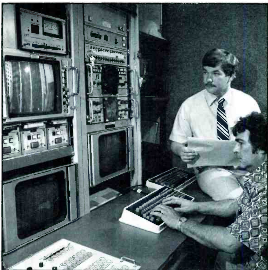
The WISH-TV automation system cuts on-air errors and improves billing. Charlie Clark (at the keyboard) demonstrates the log generating capabilities of the WISH automation system, while the author looks on.
